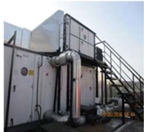
A treated fresh Air Handling Unit
