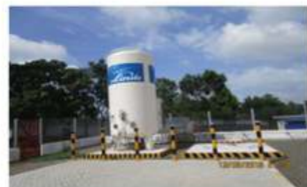
Liquid Medical Oxygen Plant
