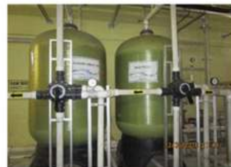
Water Filtration System
