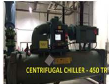
A Chiller inside the Air Conditioning Plant
